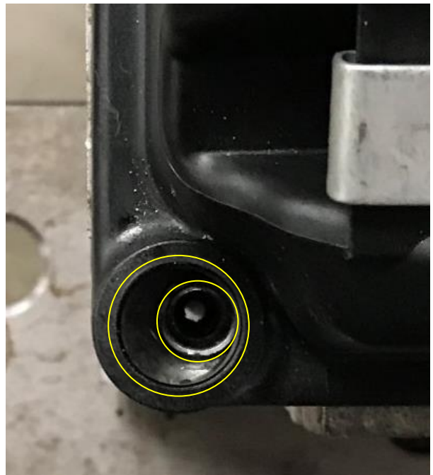
Figure 2d: Valve cover without bolt or sleeve. Housing must be forcibly deformed by installer to align fastener holes.
